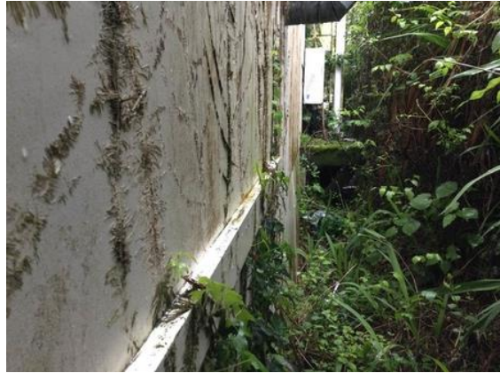
Photo is of the left side of the property facing the street. No access to assess this side but clearly not acceptable condition
