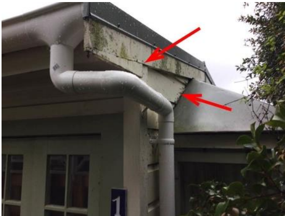
These details on the sleepout are not ideal (indicated with red arrows)
