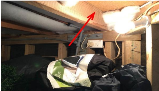
Rear side, missing piece of insulation
