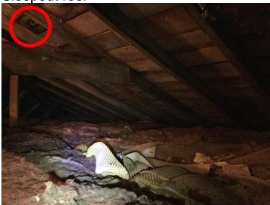
Visible moisture stains
