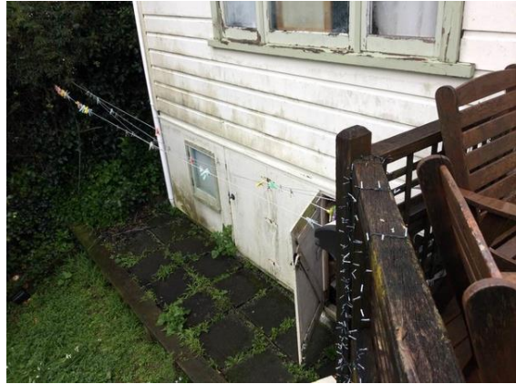
Rear side of sleepout is in bad condition
