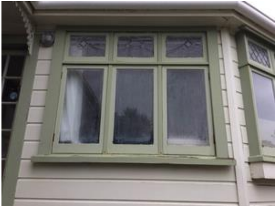
Rusted hinges on most windows
