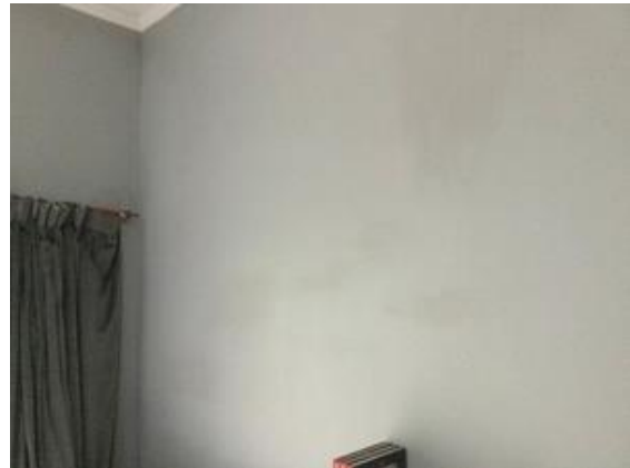
Bedroom one front right corner room has lots of markings visible
