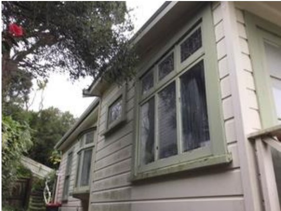
Lots of loose window glazing putty
