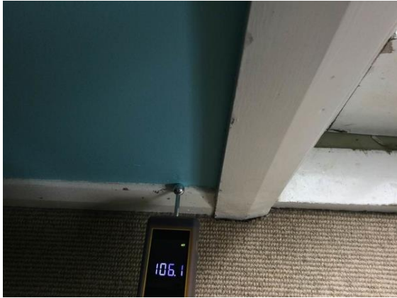
Sleepout has a high moisture reading by the door
