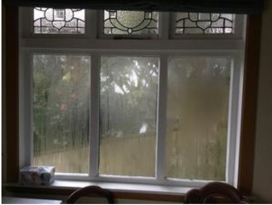
Condensation on most windows
