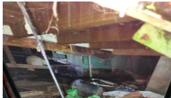
Under deck facing towards street has incomplete base board cladding
