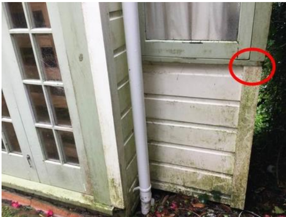
This detail on the sleepout circled in red is not ideal
