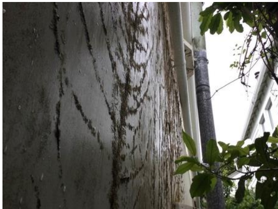
Photo is of the left side of the property facing the street. No access to assess this side but clearly not in acceptable condition
