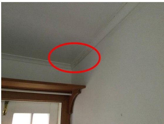
Sleepout ceiling as per photo has deterioration in this area
